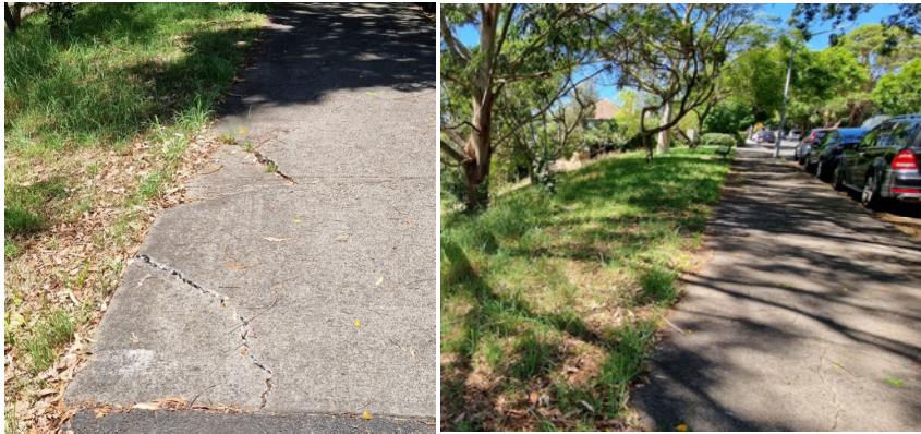
Figure 16 Tension cracks on footpath along Cranbrook Road
