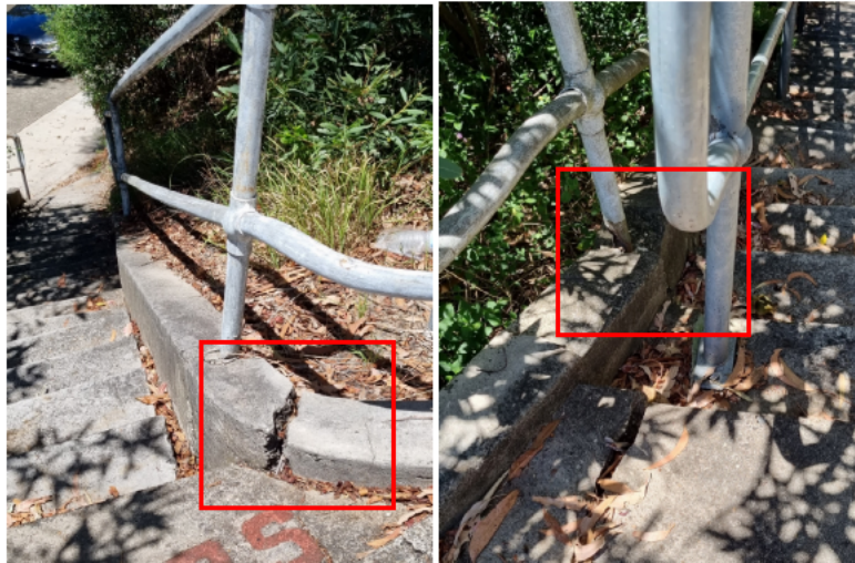
Figure 18 Cracked hand-rail kerb along an external stair.
